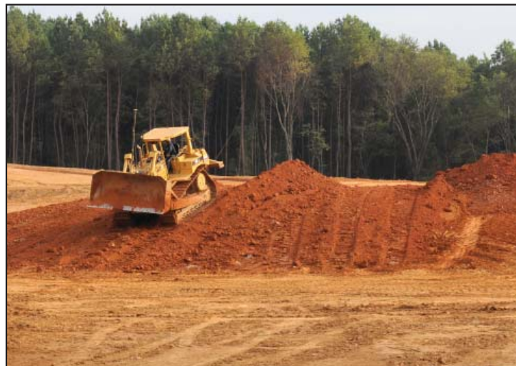
Above: A tractor drives over a dirt pile after the groundbreaking, Sept. 1. A new facility will be built there to train Airmen of the 241 st Engineering Installation Squadron.
