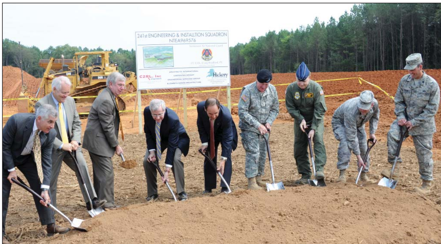
Below: Shovels are dug into the Earth to mark the beginning of construction of the 241 st EIS's new facility in Chattanooga. (Photos by Randy Harris.)
